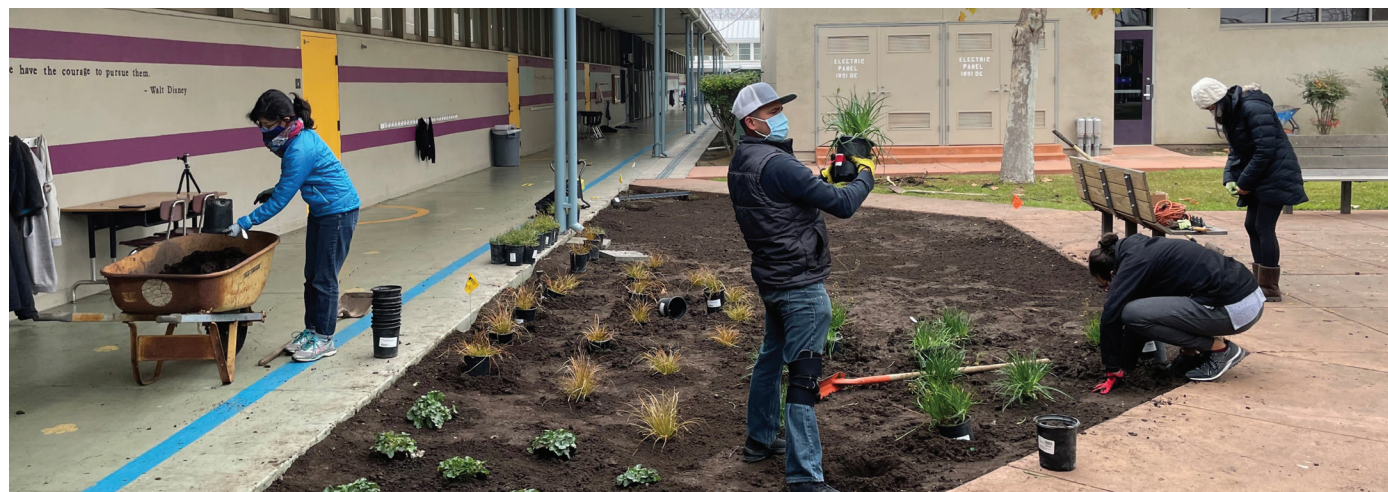
C/CAG invests in green infrastructure including at school sites throughout the County. (Image credit: C/CAG)
